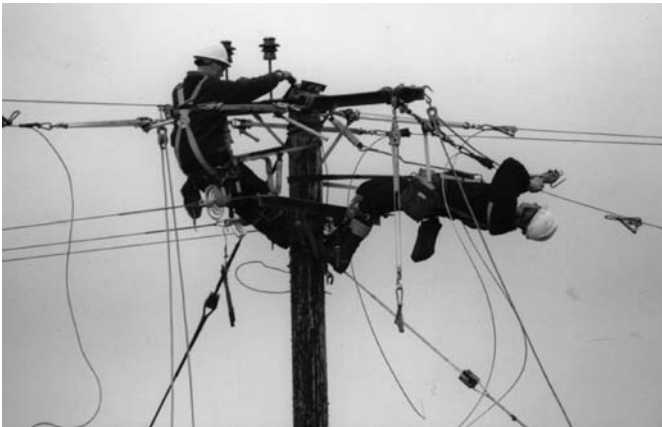
Fig. 8.5 Electricity linesmen at work. Note the extreme postures adopted. Photograph courtesy of Dr E. Wright.
